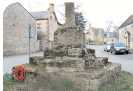
Eroded stone, base of village cross, The Hill
